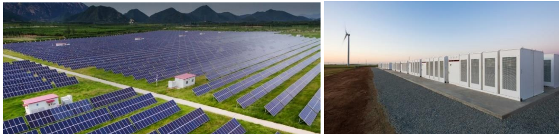
Figure 9.9. A utility scale solar farm (Source: https://recsolar.com/utility-scale-solar-solutions/ ) and the Tesla lithium battery bank, South Australia (Source: https://www.gizmodo.com.au/ ).
